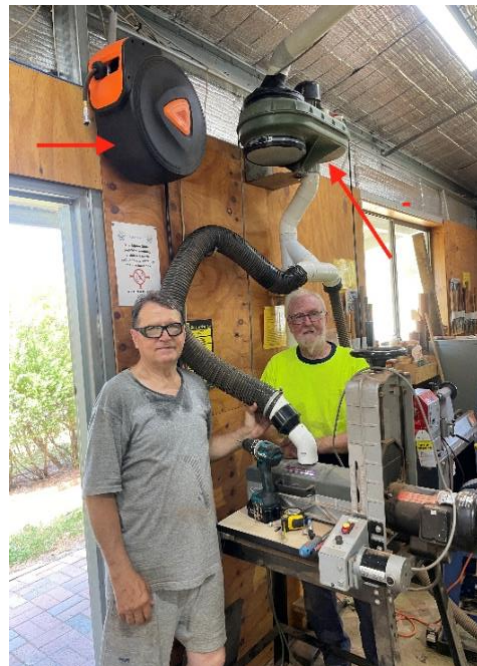
Left: Vaclav Marcak & Mal Darwent installing a compressor cable and dust extractor.
